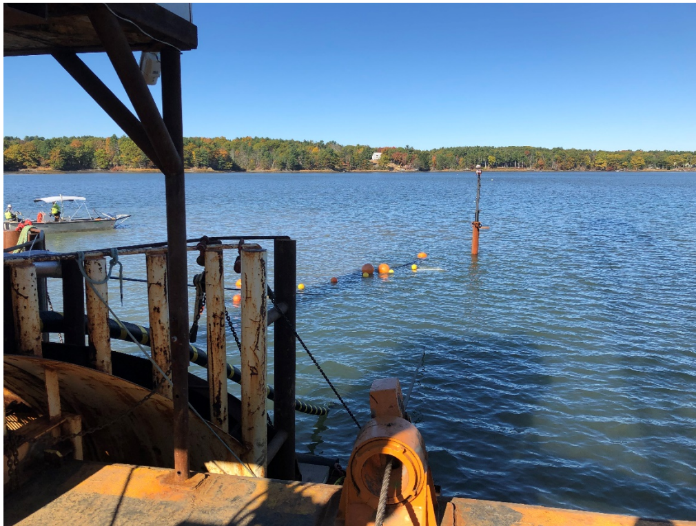
Jet sled approximately 50' of setback from cable chute and barge. Plow is located on the western side of the channel in 3 – 5 feet of water. Slightly visible, localized plume near jet plow.
